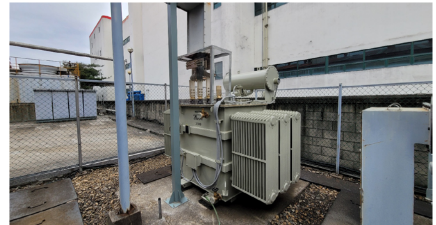
High-Efficiency Hybrid Transformer at Daejeon Plant 1
