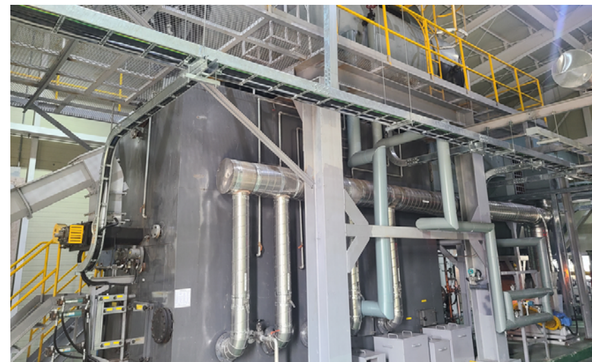
* Wood Pellet Boiler (Gwanghyewon Plant)
